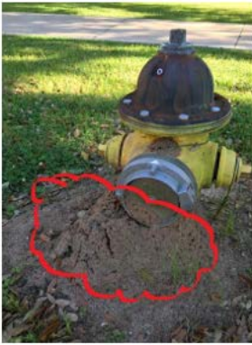
Dirt Accumulation or Ant hills
