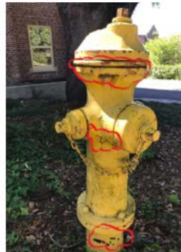
Oxidation and Cracking
