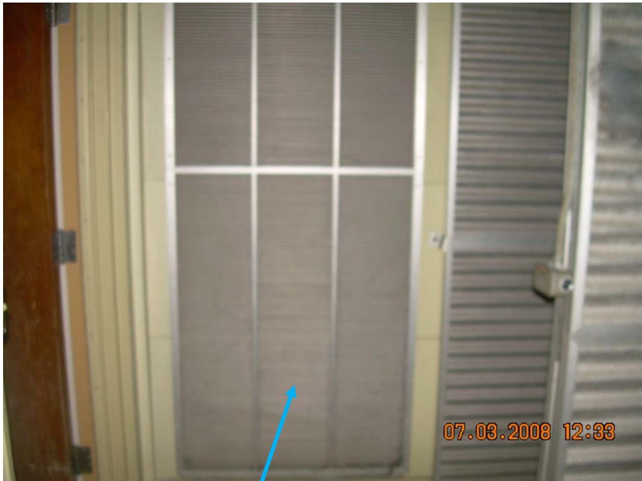
Photo 2 – Return grill – In Firing range, clean, remove wrap and dispose
